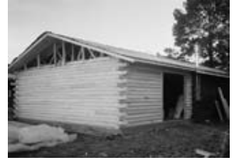
The roof is in place and the double doors are framed as construction continued on the new addition.
